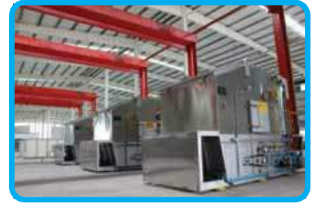
modernized battery Grid (oxygen-free) Drying equipment
