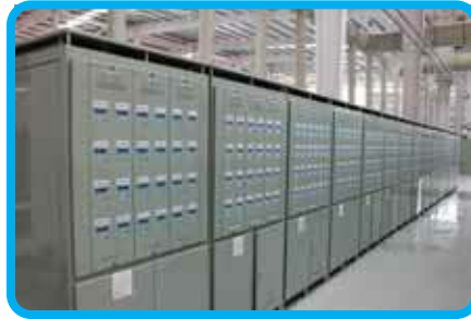
Battery charging equipment
